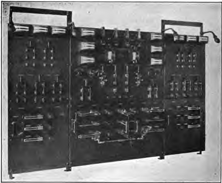
FIG. 66.—U. S. S. New Mexico : Direct Current Exciter and Auxiliary Switchboard
